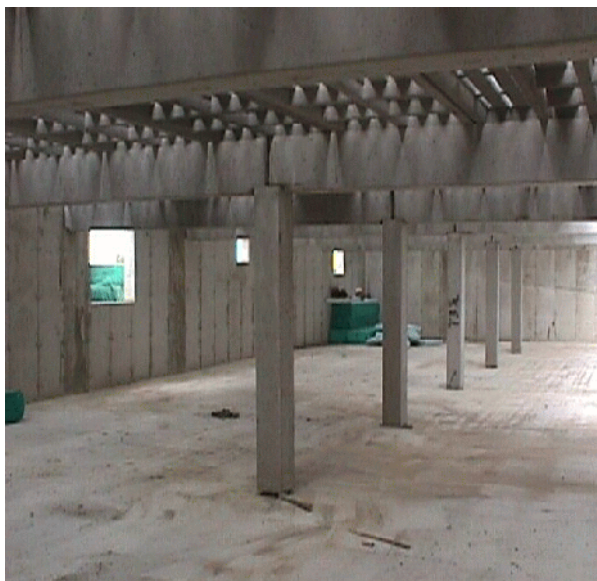
Figure 1 Downstairs in barn, during construction, showing concrete columns supporting slatted floors. Ventilation exhaust fans were installed in wall openings.
