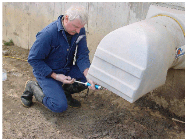
Figure 3 Malcolm MacAlpine taking a reading of the ammonia level at exhaust fan
